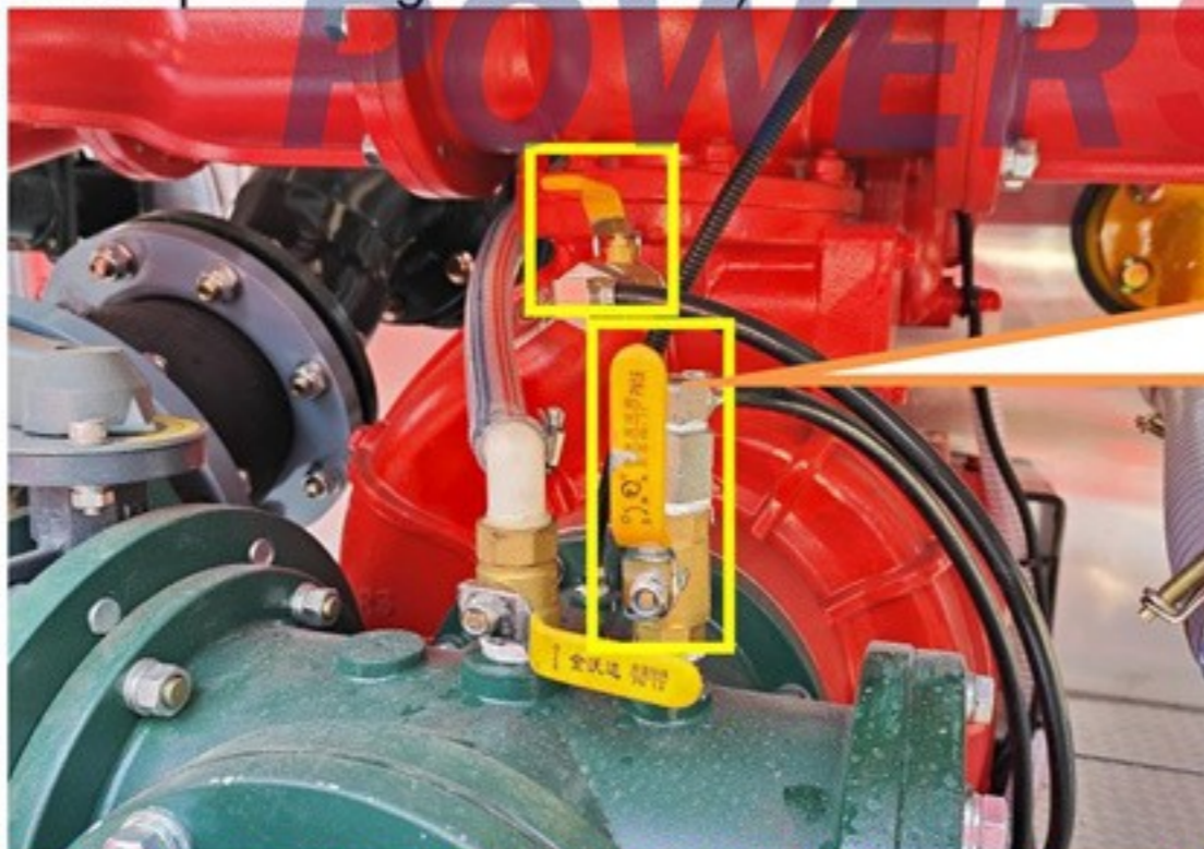
Pump & PTO Recirculating Water Valve (Cooling Switch)
